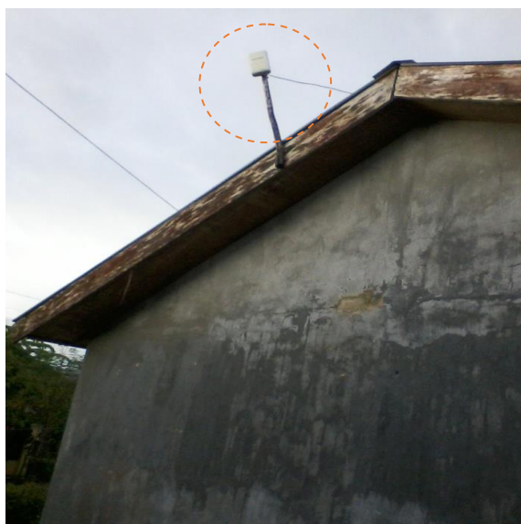
Gambar 4. Repeater Acces Point outdoor
